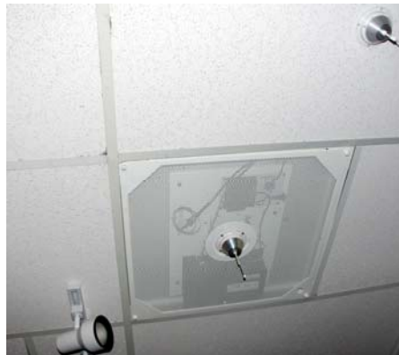
Figure 4 Typical Ceiling Enclosure Installation with Local and Remote Antennas
